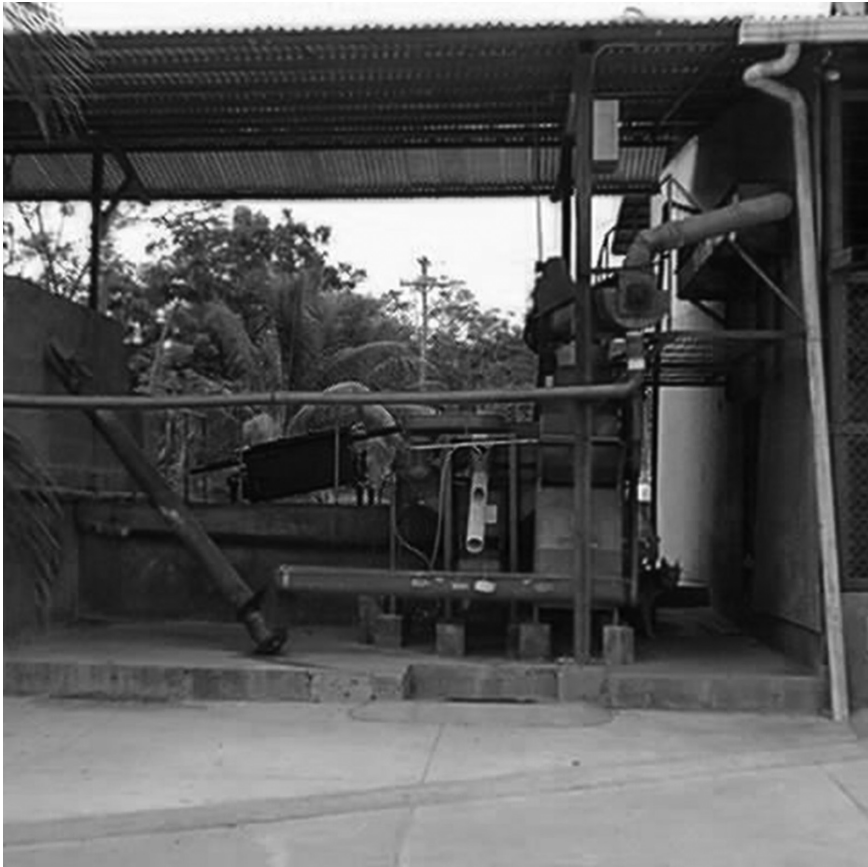
Photo 6.4 Compact ecological processing unit (UCBE) purchased to process organic coffee
